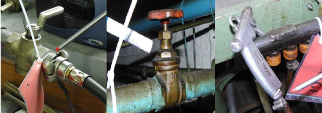
Figure 2-3 Examples of Air Leakage
